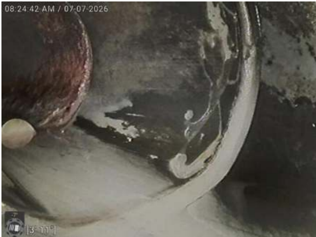
ABS TO CAST IRON TRANSITION COIN OR OTHER DEBRIS STUCK IN JOINT
