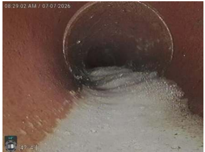
CLAY LATERAL PIPING MINOR BELLY (LOW SPOT HOLDING WATER) - ACCUMULATED SOAP SUDS
