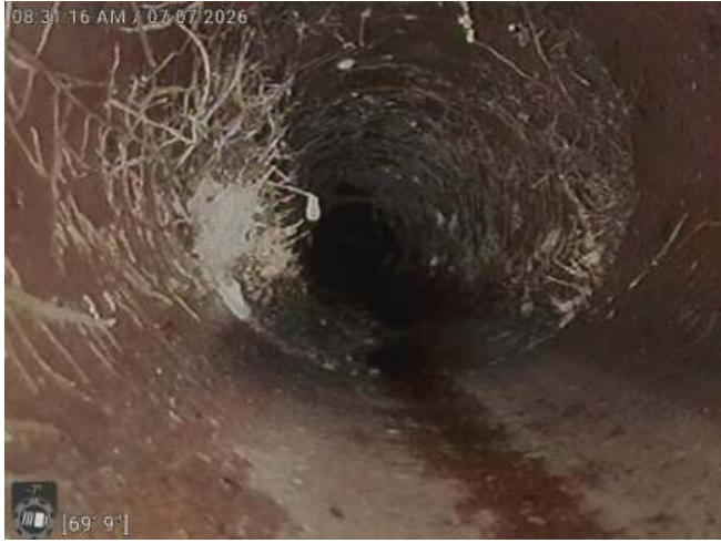
CLAY LATERAL PIPING MINOR TO MODERATE ROOT INTRUSION
