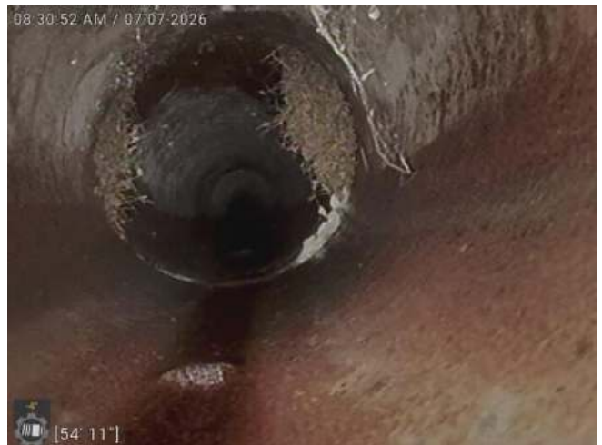
CLAY LATERAL PIPING MINOR ROOT INTRUSION AT JOINT
