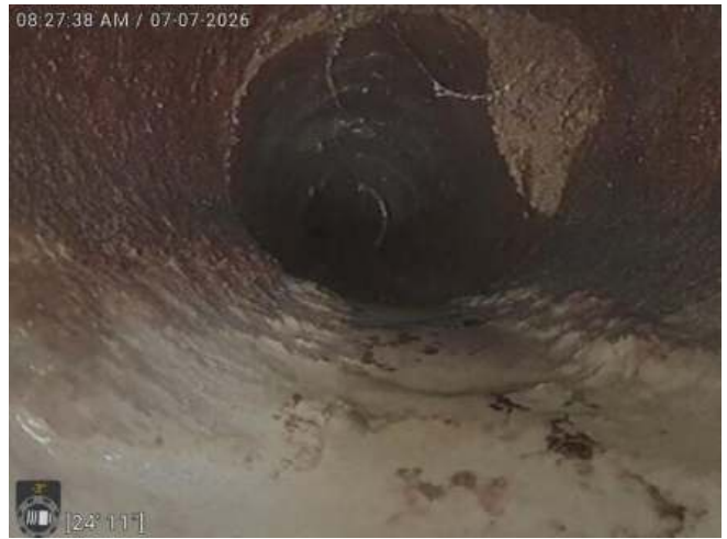
CAST IRON TO CLAY TRANSITION MINOR ROOT INTRUSION - MINOR ACCUMULATION OF SLUDGE AND SCALE
