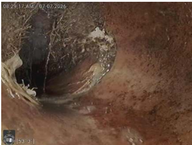
CLAY LATERAL PIPING MODERATE ROOT INTRUSION AT JOINT
