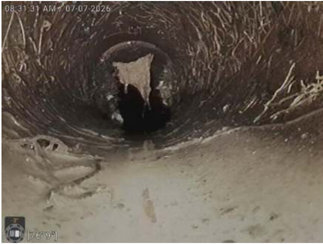
CLAY LATERAL PIPING MODERATE ROOT INTRUSION - ACCUMULATED PAPER AND WASTE
