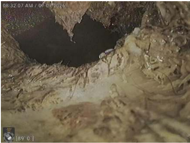
CONNECTION TO CITY MAIN SEVERE ROOT INTRUSION
