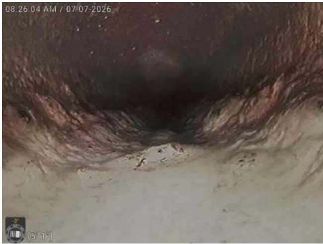
CAST IRON BUILDING DRAIN MODERATE RUST, SCALE, AND CORROSION
