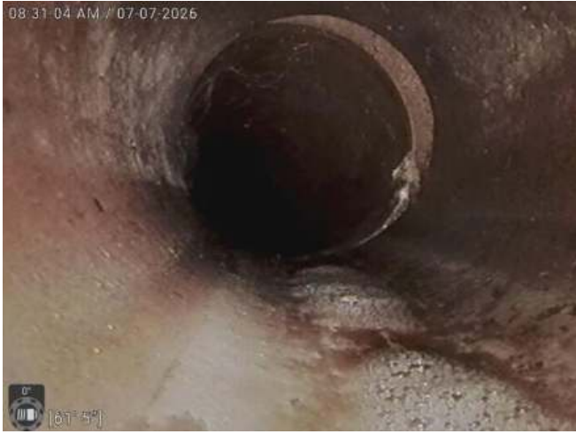
CLAY LATERAL PIPING MINOR OFFSET AT JOINT
