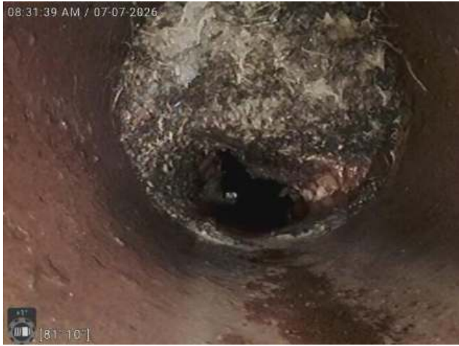
CLAY LATERAL PIPING SEVERE ROOT INTRUSION AT JOINT - NEAR COMPLETE BLOCKAGE - IMMEDIATE MAINTENANCE ADVISED TO PREVENT SEWER BACK-UP
