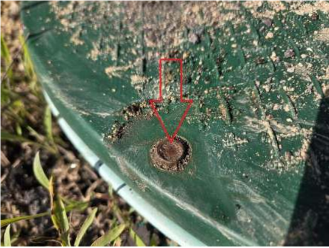
SCREWS FOR RISER LID RUSTED AND ROUNDED OUT - UNABLE TO REMOVE WITH STANDARD SOCKET - INSTALL NEW SCREWS
