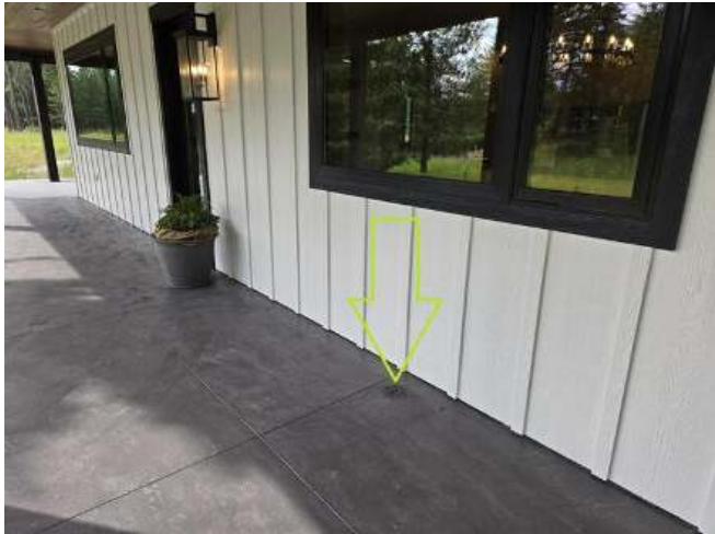
CLEANOUT LOCATION/CAMERA ACCESS MAIN HOUSE - NE PATIO
