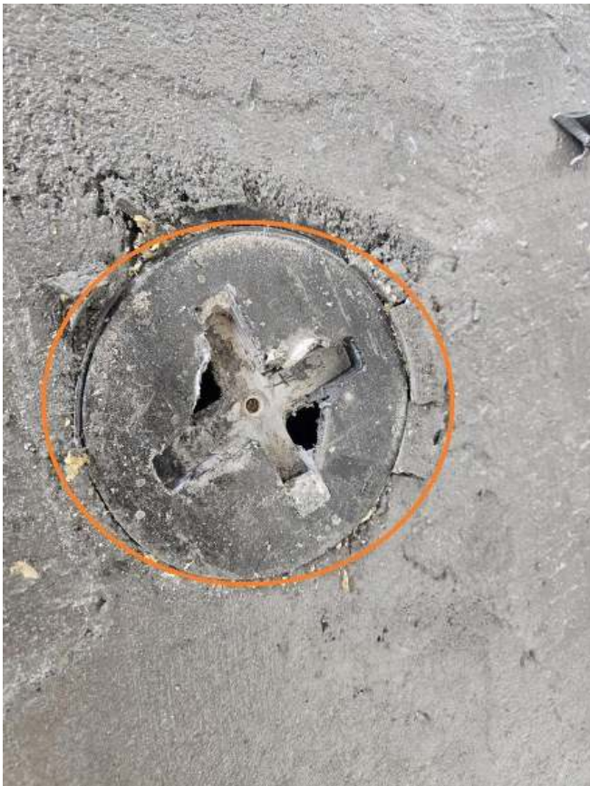
CLEANOUT PLUG CONCRETED OVER BROKE DURING REMOVAL - REPLACED WITH NEW ABS PLUG
