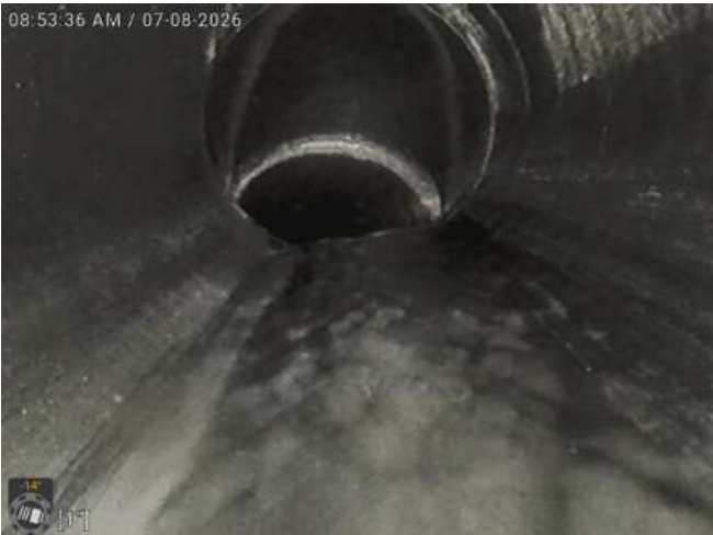
HOUSE LINE ABS PIPING - TOP OF VERTICAL ELEVATION CHNAGE
