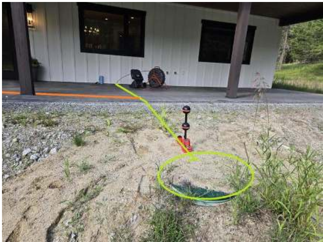
MAIN HOUSE LATERAL INLET TO SEPTIC TANK - SEPTIC TANK RISER (CIRCLED) - ORANGE LINE IS TIE-IN FROM SHOP LINE
